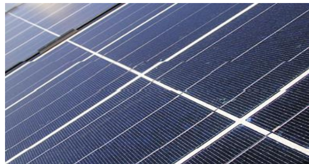
Figure 3 Solar PV panel (AER, 2008).
